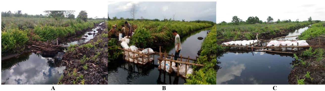
Figure 2. A. A drainage ditch in peatland before, B. During, and C. after the establishment of the water flow-dam
